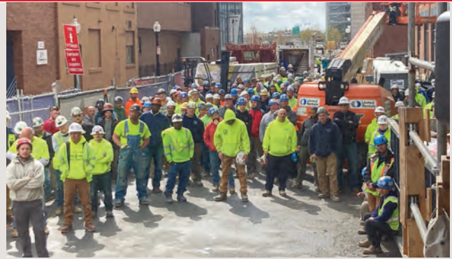
Safety Stand Down at Suffolk Construction's Harrison Albany Block Project in Boston. Photo courtesy of Mark Dellascio, Business Representative, Carpenters Local 327.
