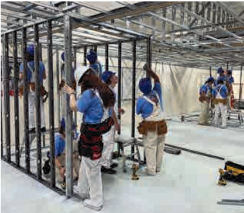
Juniors from Quincy High School took an Intro to Metal Framing class at the Boston training facility.
