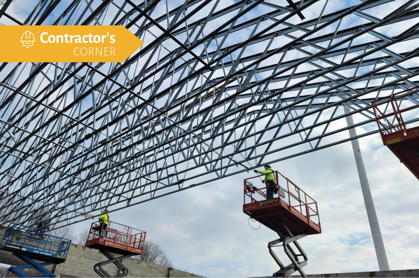
L-R Local 279 carpenters Chris Rapoli and Gregg Nott working at the Carmel Fire House Project. Photo credit Tri-State Drywall and Acoustical Inc.
