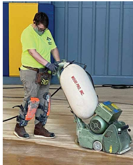
Christo Rey High School in Dorchester needed help converting old library space into a gym. They got it from apprentices and members who were happy to get back into community building! Pictured: LU 2168 Apprentice Caroline Lafferty drum stands the gym floor.
