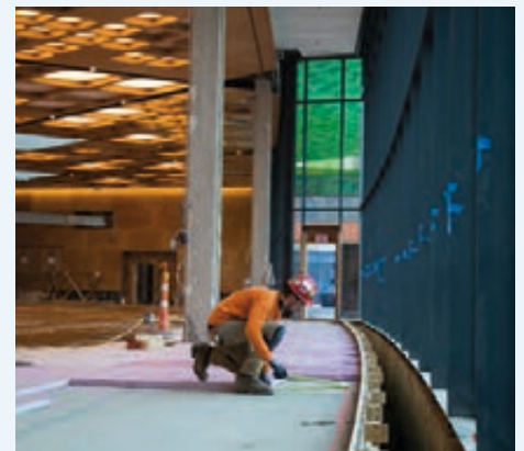
In the dining hall of the campus, Carpenters Local 336 member Corey McClure installs rigid foam in preparation for the radiant heat flooring.
