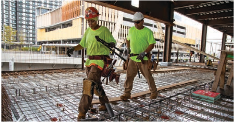
From left, Asia Tarver of Local 327 and Robert Riccio of Local 328 prepare the deck for the concrete pour.
