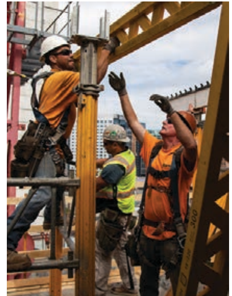
From left, Jason Linton of Local 339, Bryan Proia of Local 328 and John Conroy of Local 328 install components of the PERI formwork bracing system.
