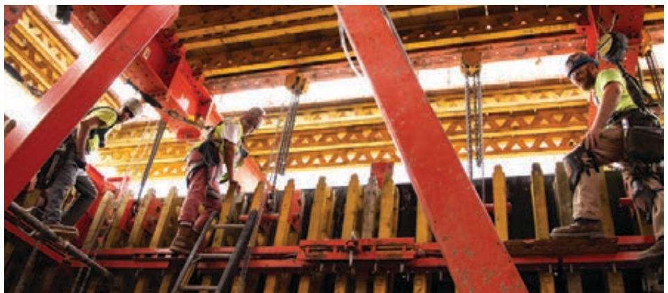
From left, Rico Cabral of Local 327, Donata Wolterding of Local 328 and Dan Crowley of Local 330 level the core wall.
